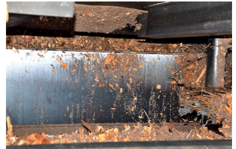
Entry point of mixed biomass into the biomass boiler.
