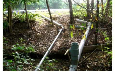
The captured biogas (methane) is transferred through pipes to the boilers where it is burnt to generate electricity.
